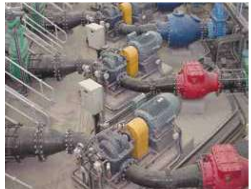
Potable Water Pump CDM400×350mm, 1,620m 3 /h, 35m, 200kW CDM350×300mm, 1,080m 3 /h, 35m, 150kW
