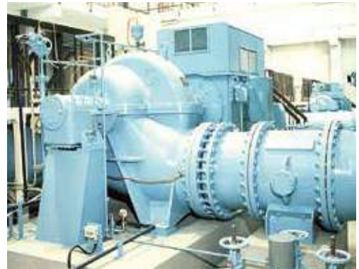
Irrigation Pump CDM800×600mm, 4,200m 3 /h, 60m, 900kW
